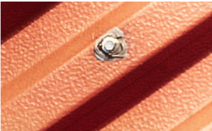
Damaged fastener on roof cladding.
